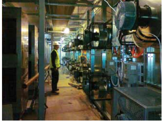
Above: Inside the purpose built containment area that houses the high volume modules (at left) and the fan wall (at right).
